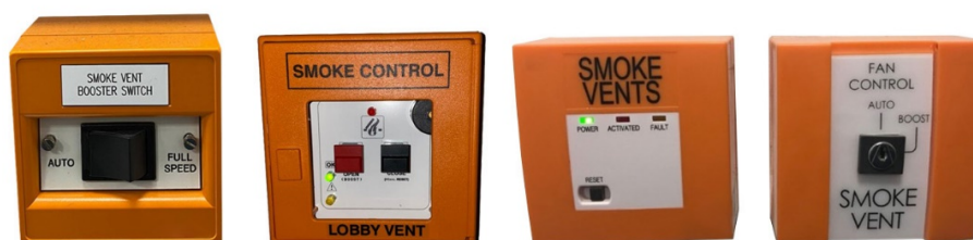
Figure 2. The design, positioning and precise function of switches can vary greatly from one supplier to another and from building to building
