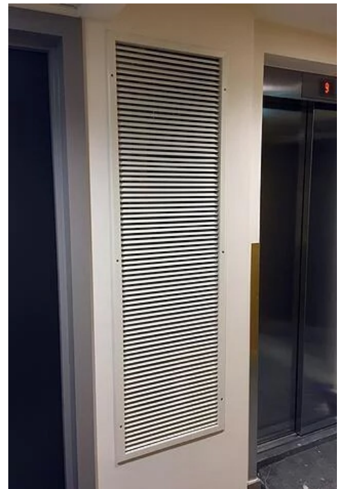
A lobby damper
