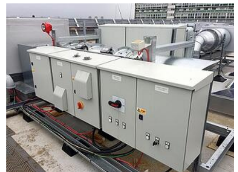
Roof-mounted fan skid and controls
