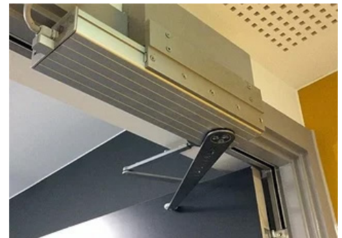
24V door opener on one of the stair doors
